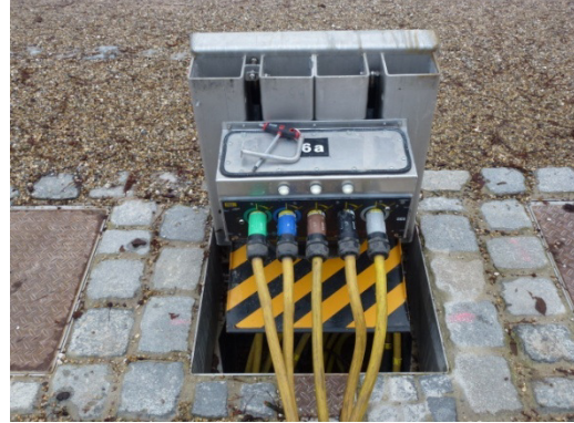
Typical shoreside power connection
