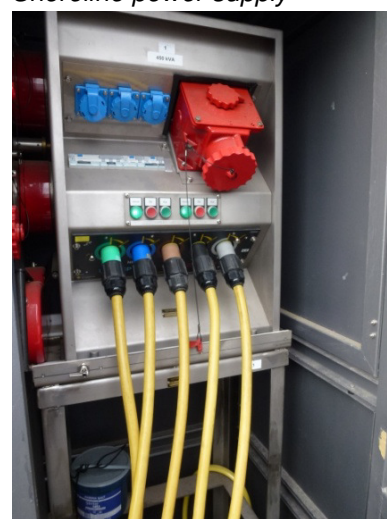
Shoreline power supply
