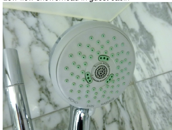
Low-flow showerhead in guest cabin
